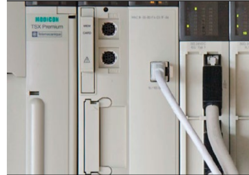
Functional testing of AMACS systems
